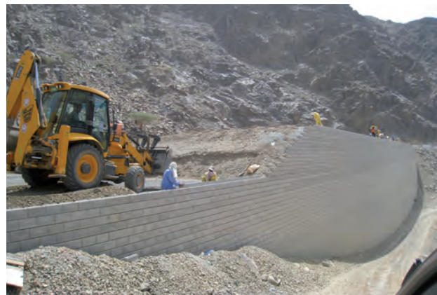
This project in the UAE demonstrates that the TensarTech TW1 Wall System can be built without cranes or propping.
