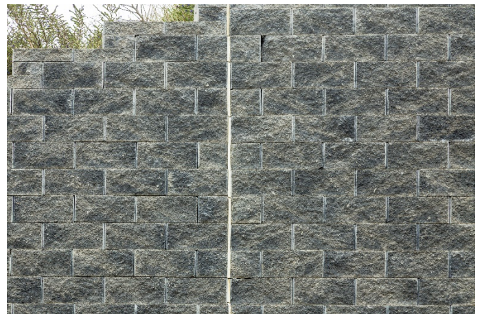
Figure 14. Slip joint post-earthquake
