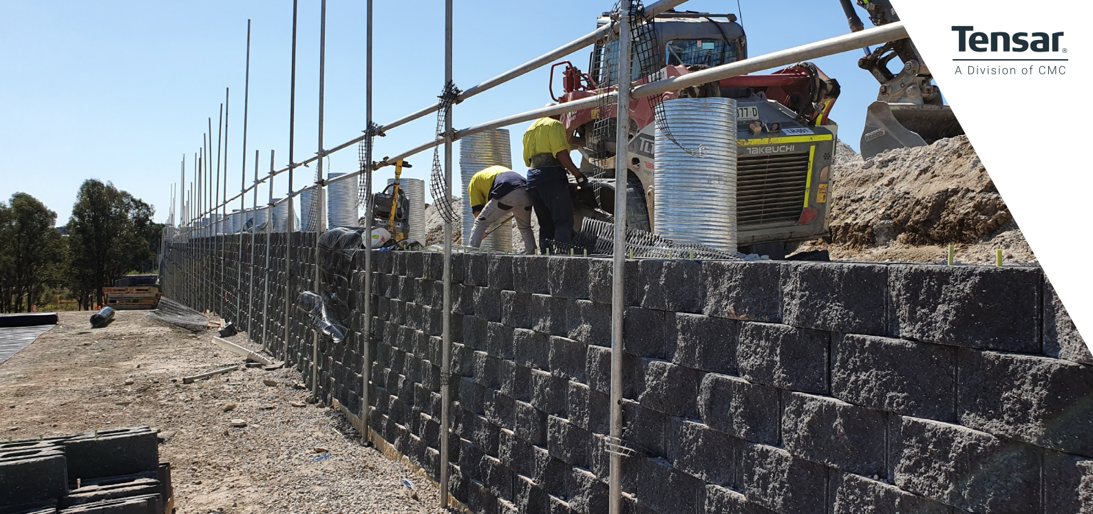
Corrugated pipes for noise wall foundations were installed close to the wall face, surrounded by Tensor RE uniaxial geogrids
